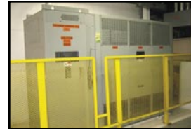
FEDERAL PACIFIC 600-AMP. 5KV MAX. SWITCHGEAR
