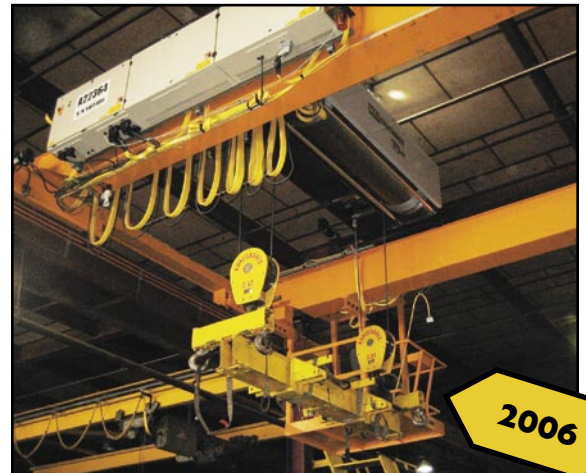
KONE 5-TON OVERHEAD DOUBLE-HOOK BRIDGE CRANE
