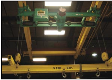
P&H 5-TON CAPACITY DOUBLE HOOK BRIDGE CRANE
