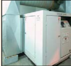
GARDNER-DENVER 75 HP rotary screw air compressor
